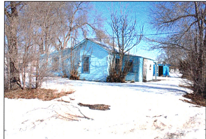
Photo 1: Aged and dilapidated buildings provide evidence for substandard determination in Site 1.
