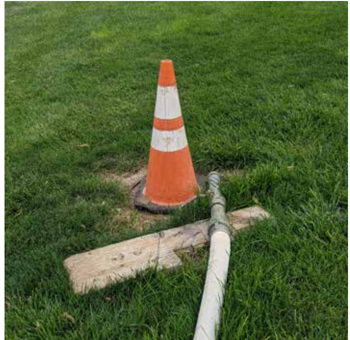
Existing sprinkler system on northeastern portion of site.
