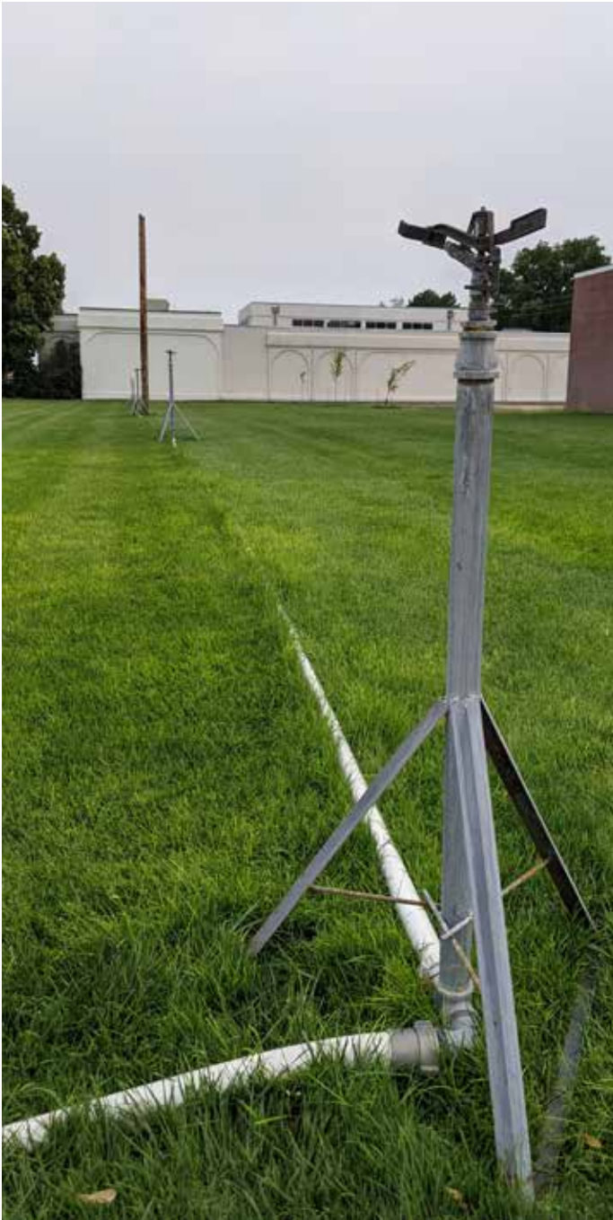
Existing sprinkler system on northeastern portion of site.
